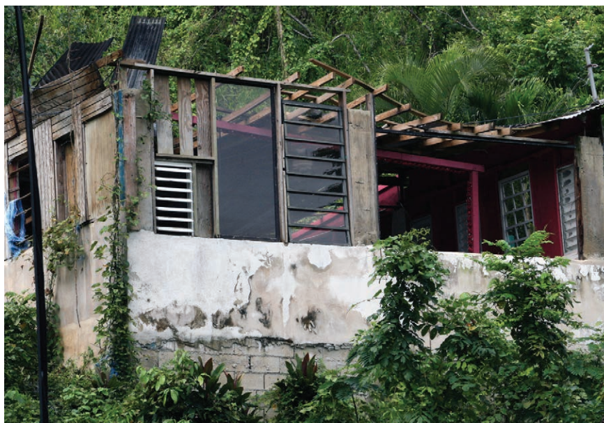
The force of Hurricane Maria's winds blew the roofs off many homes on the island. The fact that this home does not have one of the blue tarps supplied by FEMA indicates it was likely abandoned after the storm.
