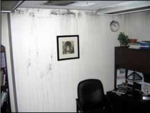
Soot damage in Susan Dow's office
