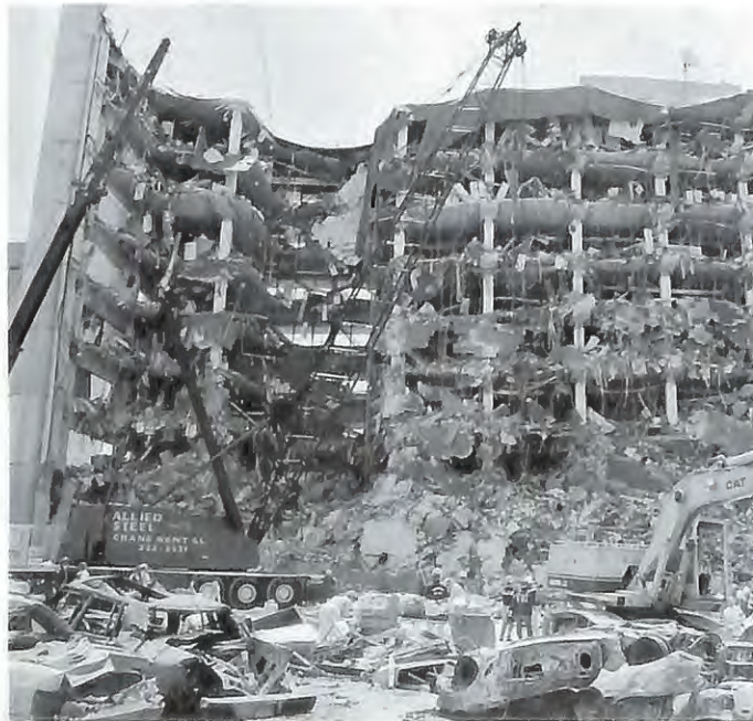
Heavy equipment is used to remove debris from the front of the Alfred P. Murrah Federal Building in downtown Oklahoma City Friday, April 21, 1995. (AP Photo/David Glass)
